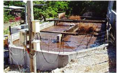
Oxidation ditch-type batch activated sludge treatment tank
